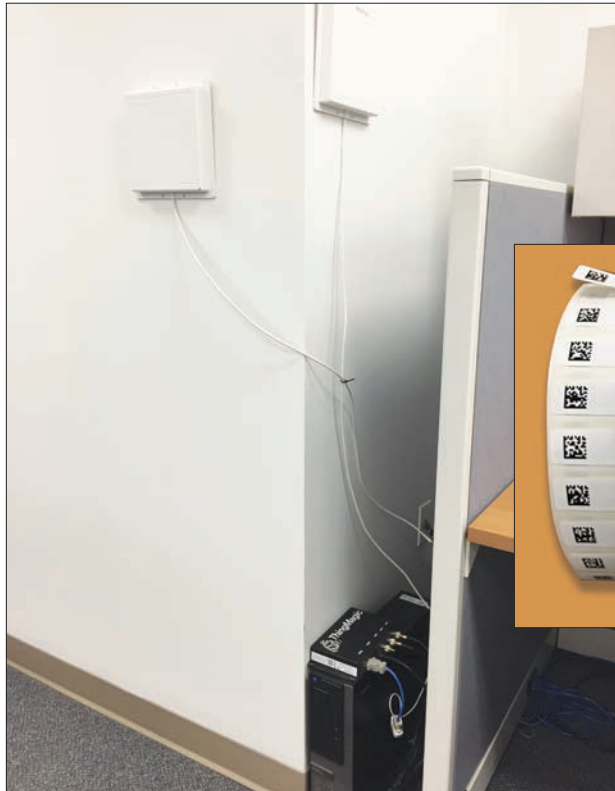
The readers can see tags located up to approximately 20 feet from the chokepoints. Inset: Each RFID tag is printed and pre-encoded with a unique identification number.
